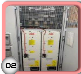
Open Cabinet with Fuses on Top
