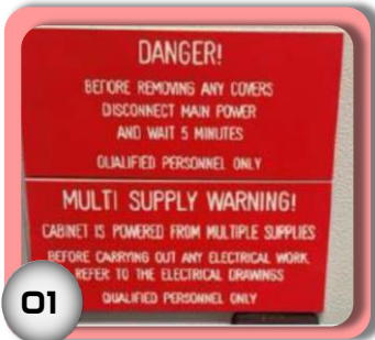
Signage on Cabinet Door
