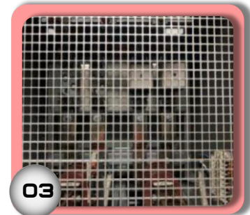
Fuses Behind Protective mesh
