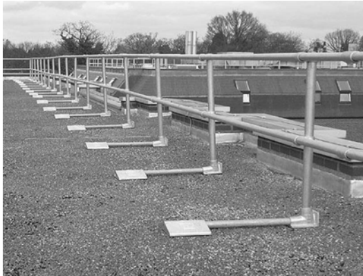
FIGURE 27.8 Guardrail system near the edge of a roof.
