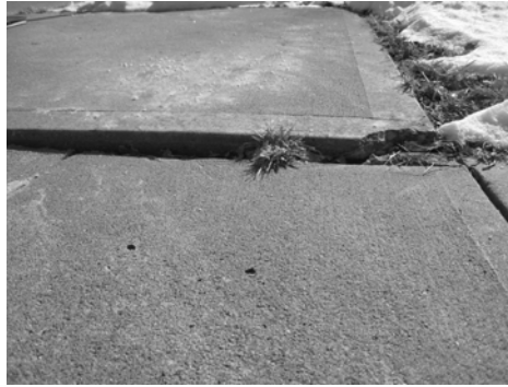
FIGURE 19.2 Unmarked sidewalk tripping hazard (unevenness exceeding \frac{1}{4} in.). (Courtesy of Chris Janson.)
