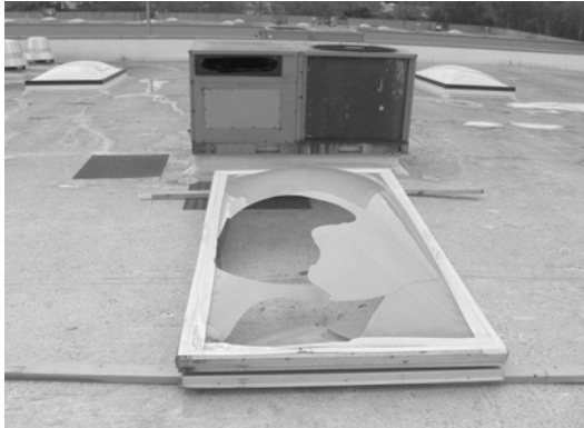
FIGURE 27.1 Skylight on a roof that had a fall through.
