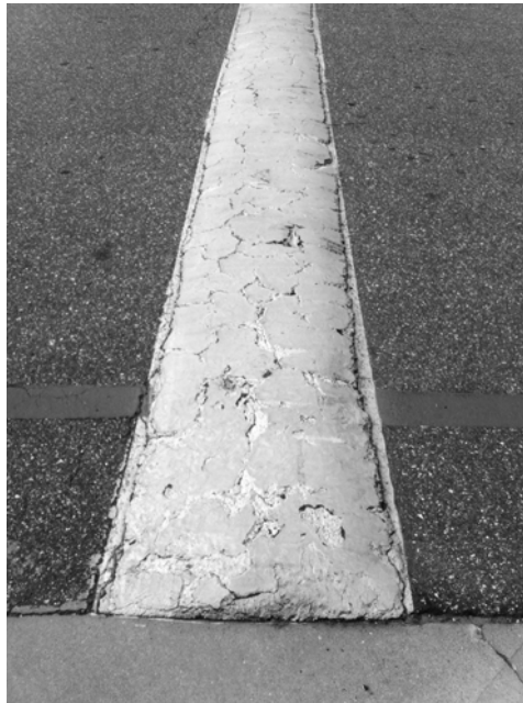
FIGURE 19.8 This speed bump is well marked, although it is in deteriorating condition.
