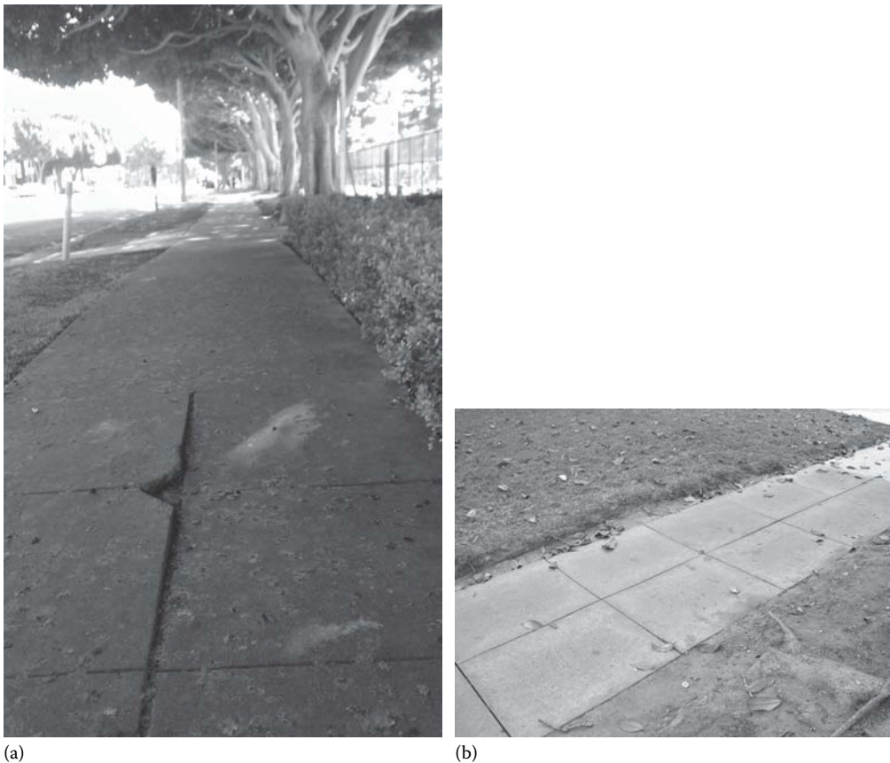
FIGURE 19.3 Side-by-side comparison of the original concrete sidewalk (a) and a recycled plastic replacement (b). (Courtesy of TERRECON, Inc. www.terrecon.com .)
